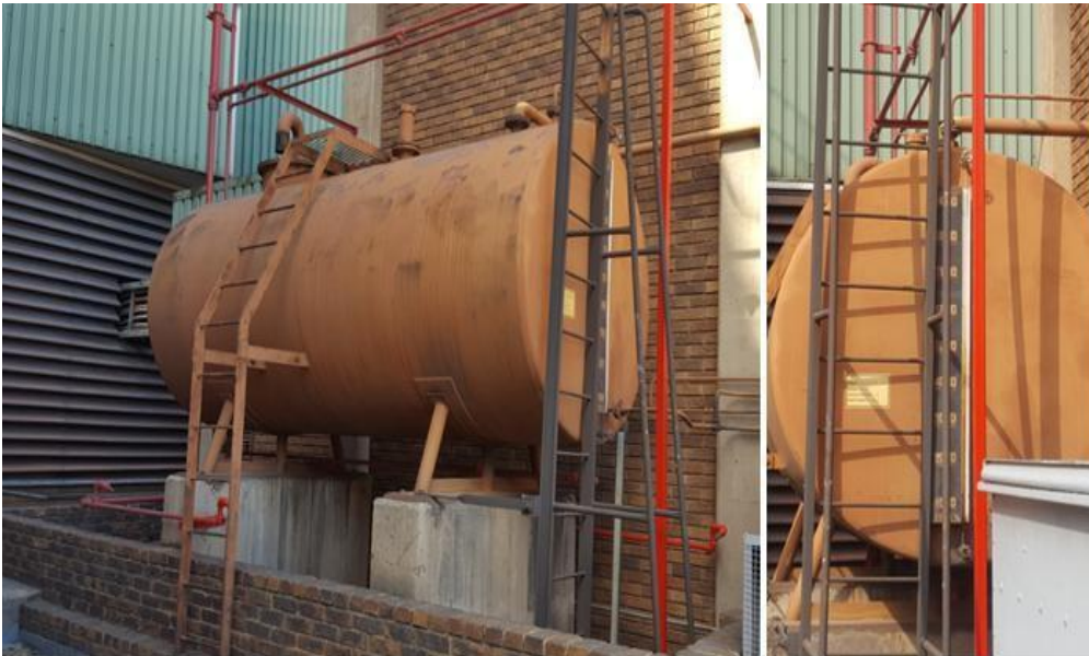
Figure 8: Diesel Storage Tank and Level Indication
