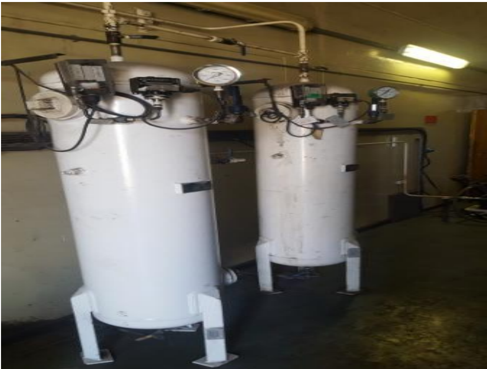
Figure 5: Existing Air Receivers
