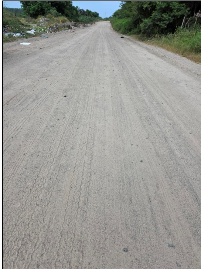
Photo 2: Current condition of the centre of the road.
