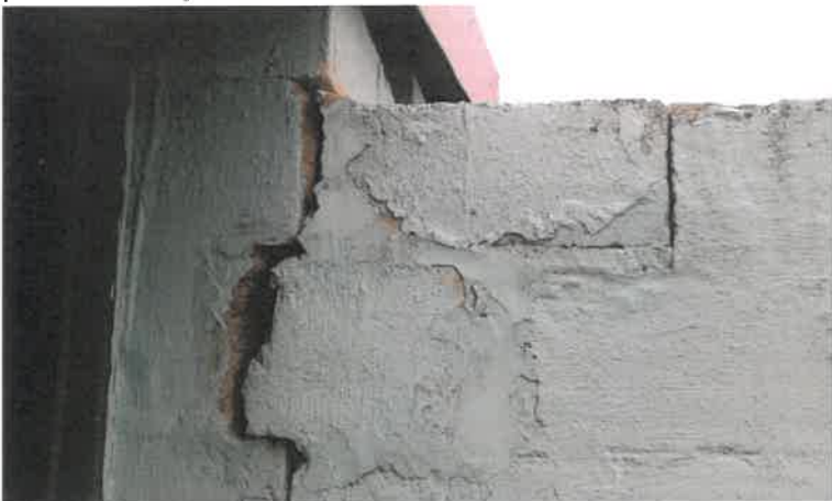
Figure 2: Specific Defects (cracked walls)
