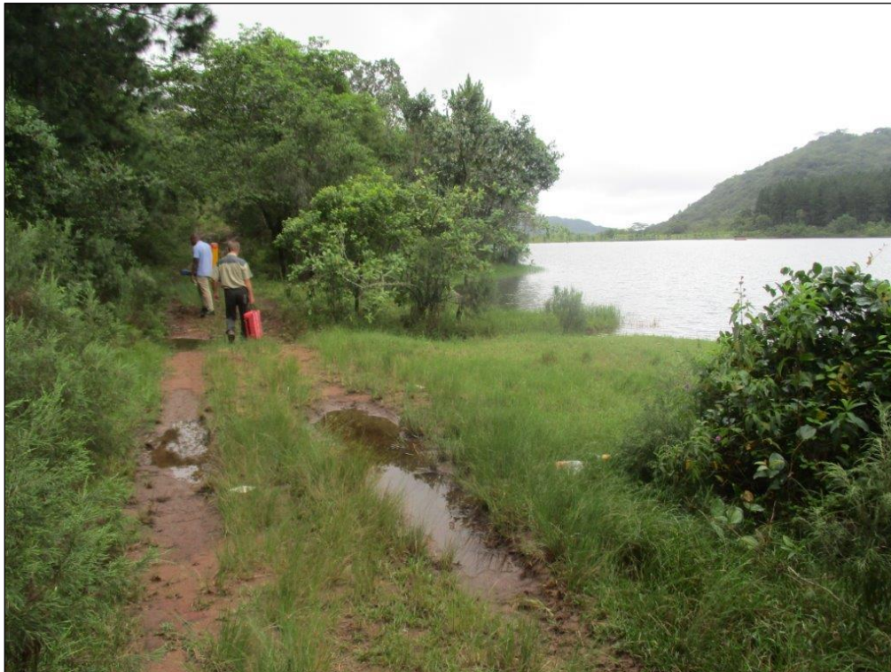
Figure 13: Condition of access road
