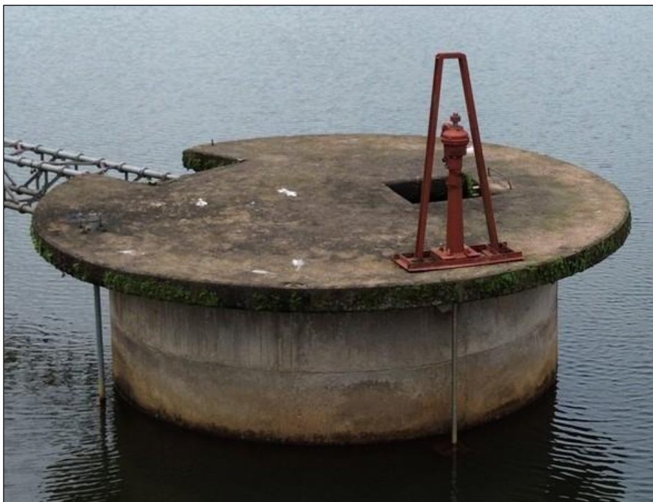
Figure 9: Intake tower sluice gate controls
