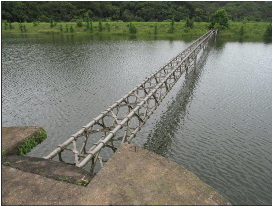
Figure 11: Remains of old walkway
