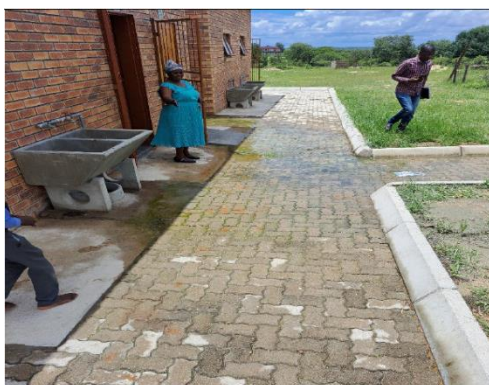
Inadequate drainage on pavement caused by groundwater
