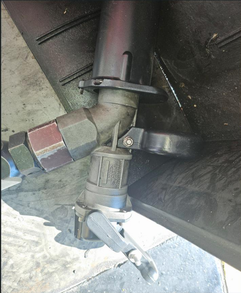
Outflow Wiggins Nozzle - Pic 1.jpg
