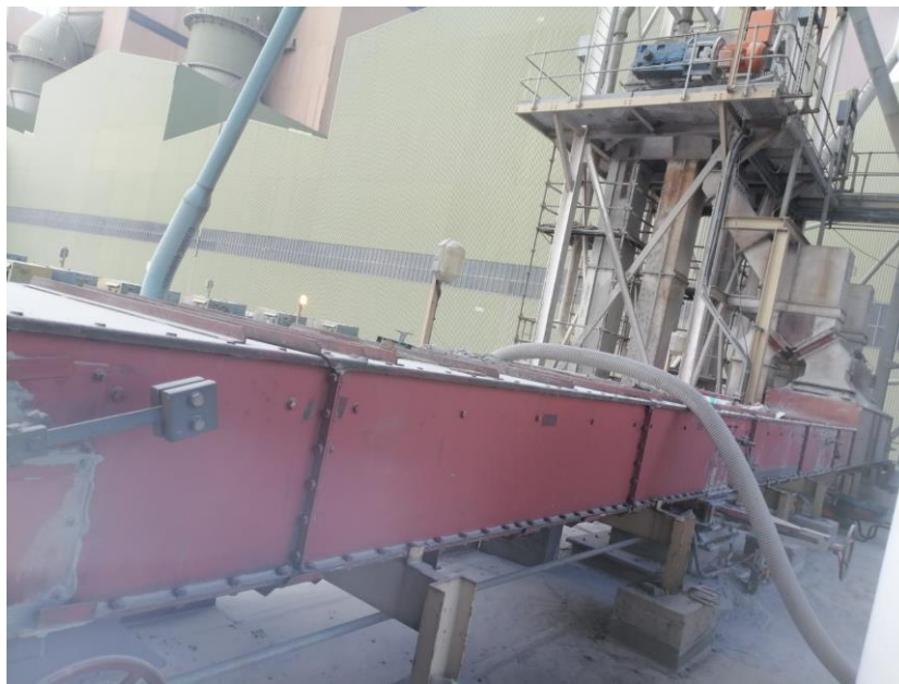
Figure 10: Bunker Top Conveyor System
