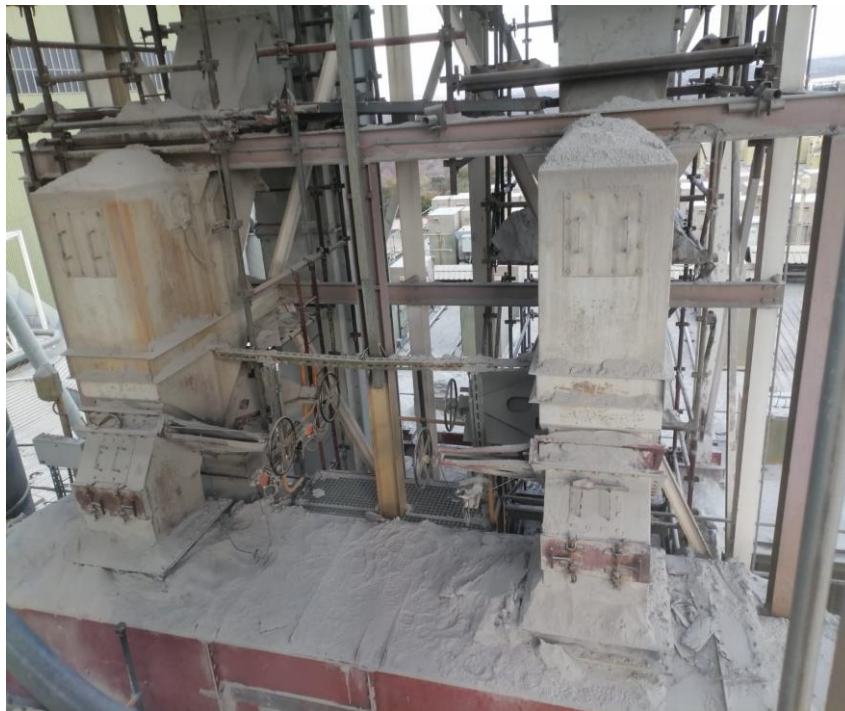
Figure 11: Slide gates on Bucket Elevator routes
