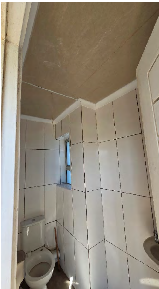
WC CEILING & LIGHTS INCOMPLETE REPAINT TIMBER DOORS SEAL AROUND WINDOW FRAMES & REVEALS WEEDS IN PAVING
