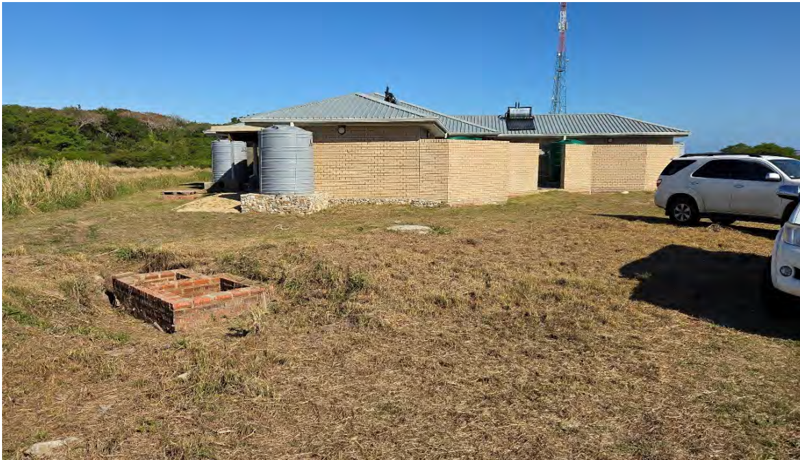
MISSING LIDS ON 2 RAINWATER TANKS & MISSING TAP ON 1 TANK
