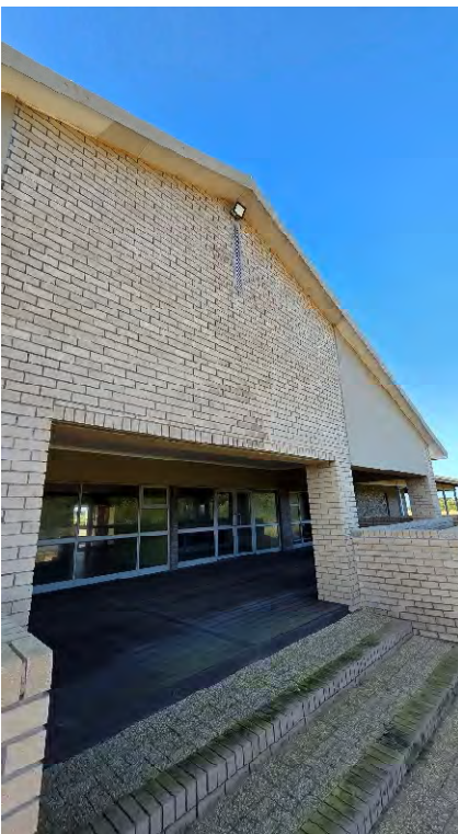
INCOMPLETE PAINTING TO EAVES BARGEBOARD
