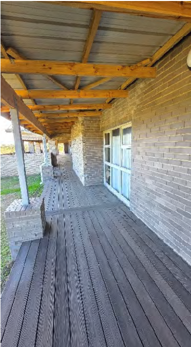
LAMINATED BEAMS SHOWING SIGNS OF WEATHERING NO WINDOW & DOOR FRAME SEALANT IN REVEALS
