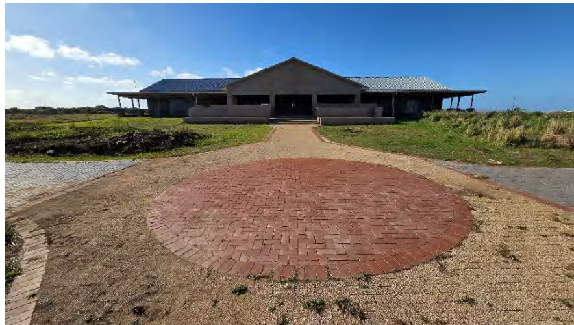
RUSTING STEEL BRACKETS, NUTS & BOLTS ON VERANDAH WEEDS IN PAVING MISSING EAVES CEILING TO LEFT OF GABLE DAMAGED FASCIA TO RIGHT OF GABLE REPAINT ALL EAVES & BARGEBOARDS NO HANDRAILS ON STEPS & NO GRAB RAILS ON RAMP CONCRETE VISIBLE ABOVE GROUND ON LEFT GABLE (WEST)
