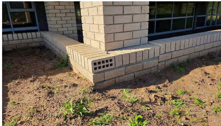
UNACCEPTABLE BRICKWORK ON PLANTER BRICK ROLLER COURSE NOT MITRED ON CORNERS MISSING CEILING BOARDS ABOVE FIRE EXIT ON WEST GABLE HOLES IN WINDOW CILL BRICK SIDES NOT FILLED
