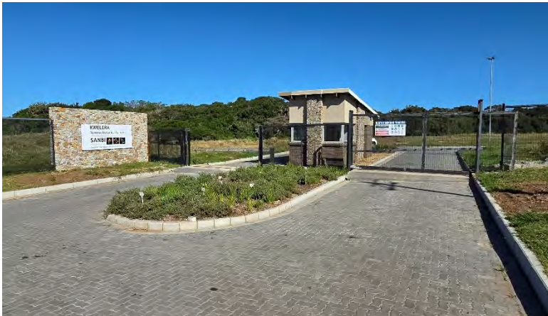
SLIDING GATES, TRACKS & SOME FENCE PANELS RUSTING CONCRETE SPILL ON FENCE TO RIGHT OF OUTGOING LANE
