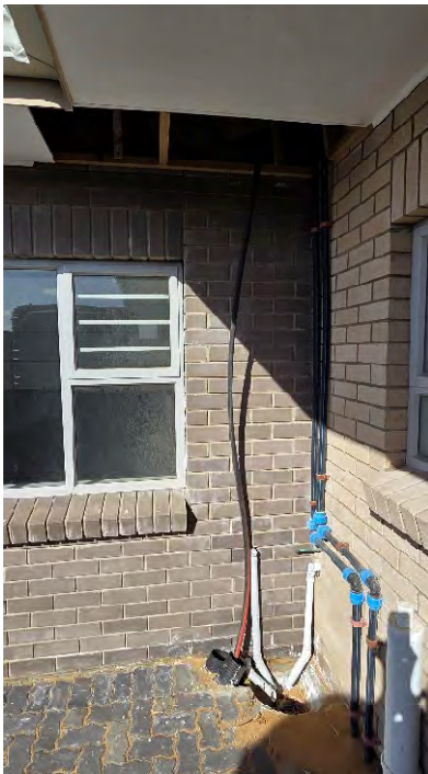
INCOMPLETE ELECTRICAL SLEEVE & CABLE & LOCATED RIGHT NEXT TO GULLEY MISSING EAVES CEILING BOARD
