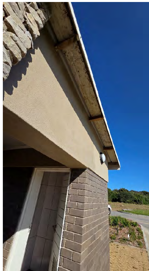
DIRTY ROOF SHEETS ONLY HALF OF DAMAGED GATEHOUSE ROOF SHEETS REPLACED & HALF GREEN & HALF GREY. TO BE REPLACED COMPLETE
