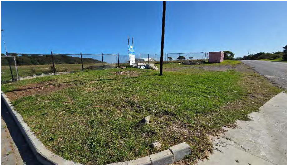
DAMAGED PROJECT NOTICE BOARD CONTAINERS & BUILDING MATERIALS LEFT UNPROTECTED UNACCEPTABLE FENCE RE-INSTATEMENT AT TEMPORARY SITE ACCESS NEXT TO WATER RESERVOIR
