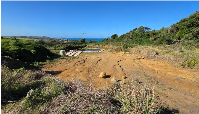
EROSION & INCOMPLETE SEWER TREATMENT PLANT NO FENCING AROUND SEWER POND
