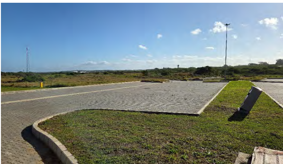
INCOMPLETE GRAVEL PORTION OF PARKING & ACCESS ROAD TO STAFF FACILITY PIPE ROAD CROSSING NOT FUNCTIONING PROPERLY WEEDS IN PAVING ELECTRICAL KIOSK LEANING OVER GENERAL SITE LEVELLING AT BUILDINGS INCOMPLETE GRAVEL PARKING AREA AT STAFF FACILITY NOT DONE
