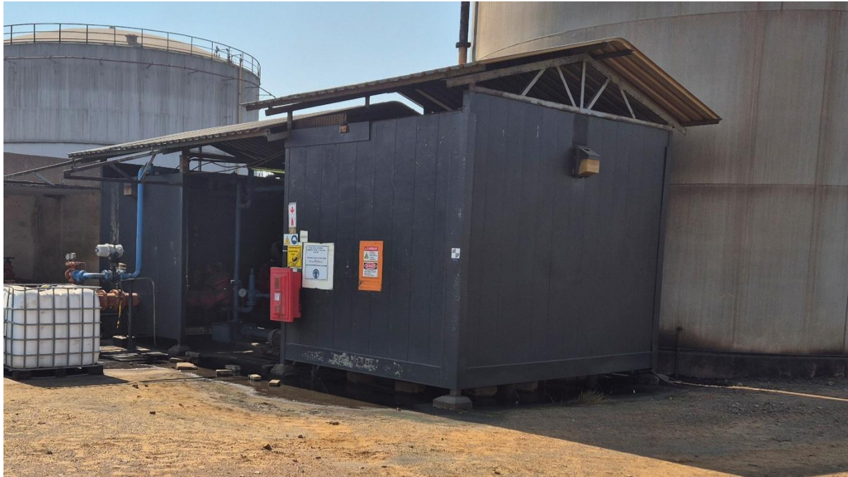
Figure 4: The pump house with existing features and equipment
