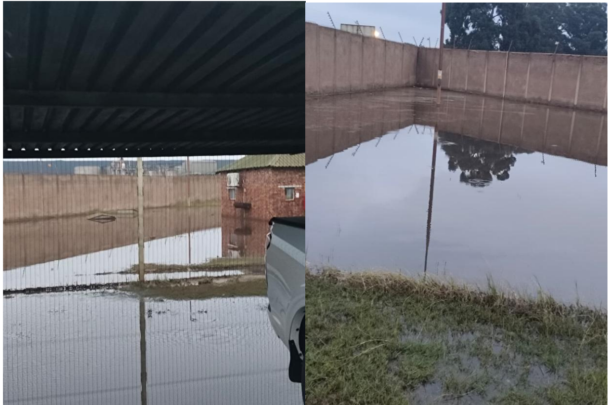
Figure 8: The figures above display the extent of flooding in the south east corner of the site and along the southern perimeter of the site.
