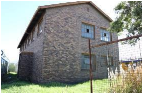
Figure 8: Old Mess Facility (which has been rehabilitated to house Gibela personnel temporarily)
