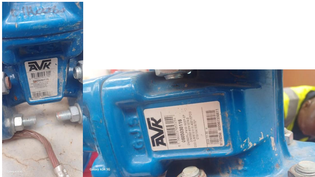
Jockey Pump Suction and discharge valves
