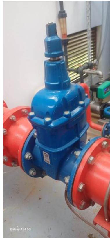
Electric Pumps Suction Valve
