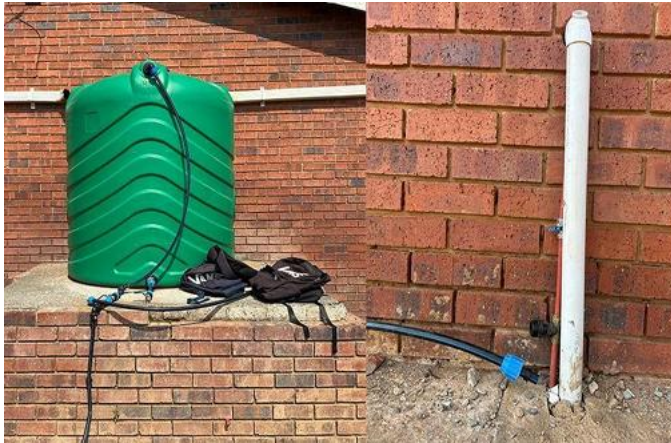
Figure 3: The water tank pipework should be relocated behind the tank to minimize exposure to tampering
