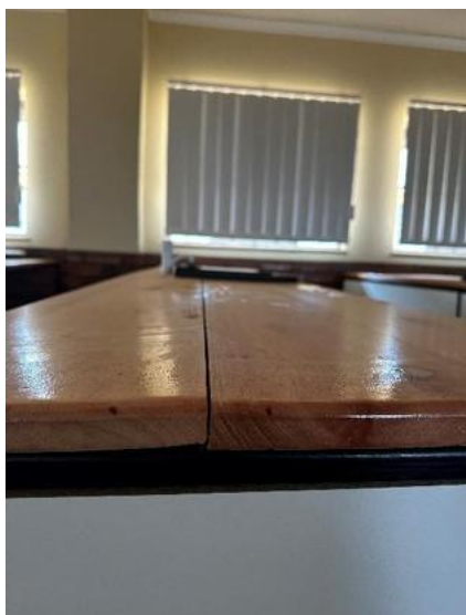
Figure 2: The cracked laboratory desktop should be replaced
