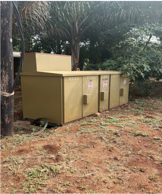
Start Point: Mini-substation Bourhill St. Coordinates: -25.441017, 31.948534
