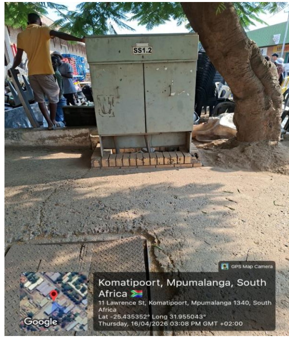
Connection Point: MP Cash & Carry Coordinates: -25.435377, 31.955045
