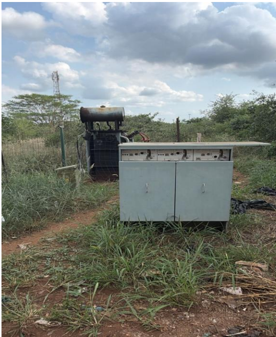
Start Point: Transformer Rissik Street Coordinates: -25.434672, 31.953523.
