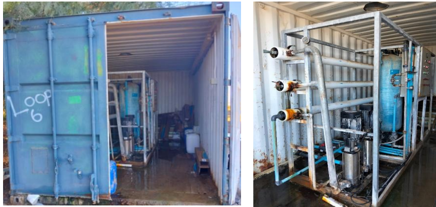
Fig. 1 Typical Reverse Osmosis plant in shipping container
