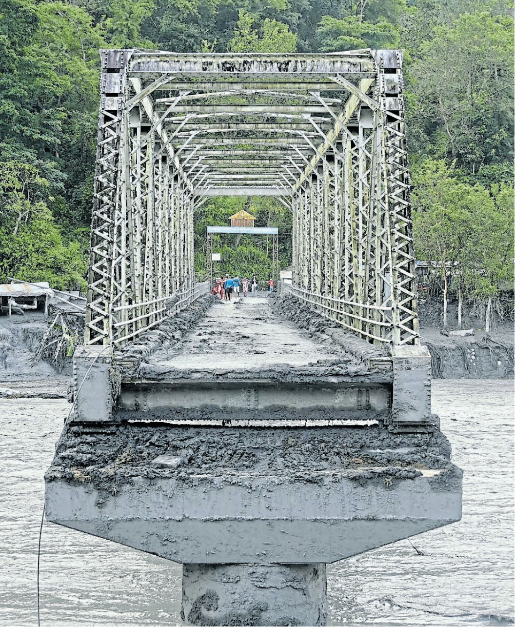
People look at the Budhi Gandaki river on a damaged bridge connecting Nepal’s Dhading district and Gorkha district, in the aftermath of a flash flood caused by a dry landslide Picture: PRAKASH MATHEMA/AFP
