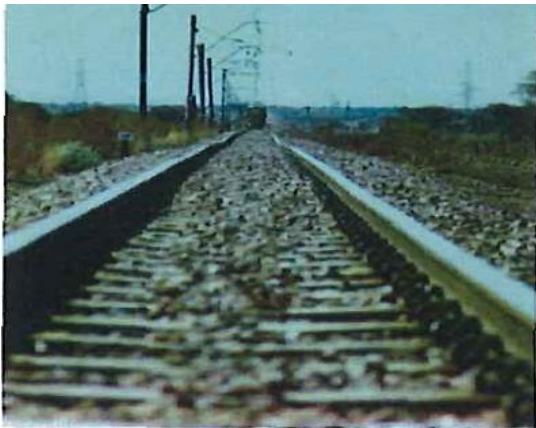
Figure 228: Vertical Alignment Defect Clearly Visible before Tamping
