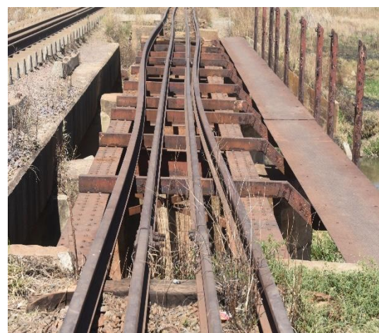
Fig 2.4: Stolen sleepers at Stretford – Residencia bridge
