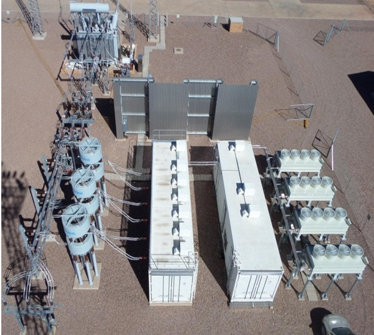
Figure 1: Aerial view of the 11 kV STATCOM equipment at Garona Substation
