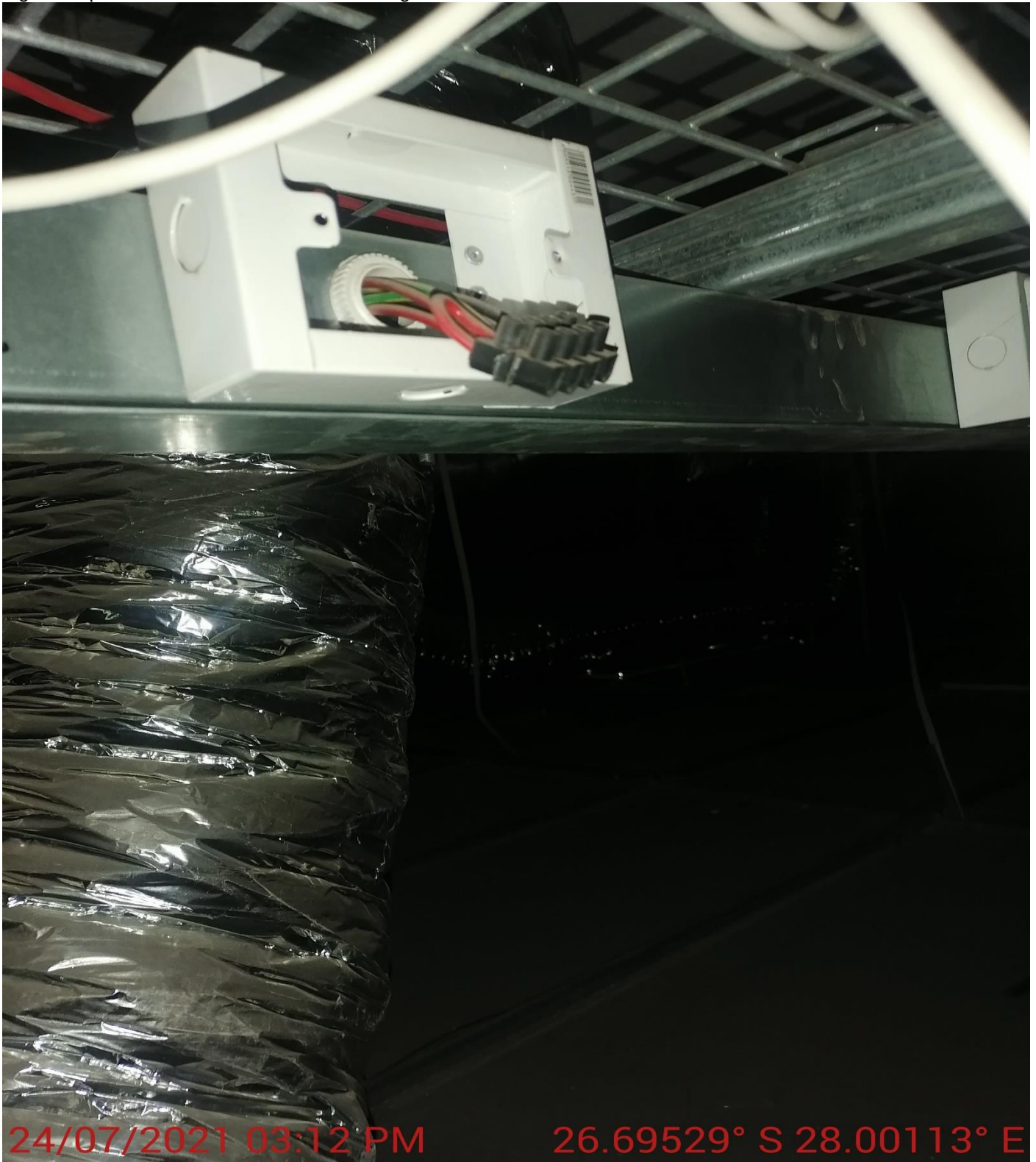
Fig 19 - Open Junction Boxes inside the ceiling void
