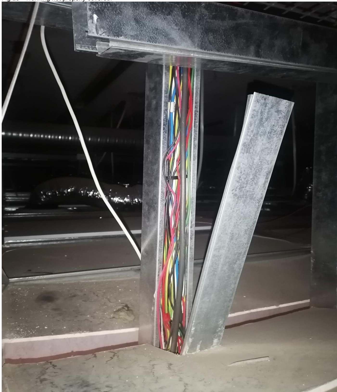
Fig 15 - Trunking not properly covered.
