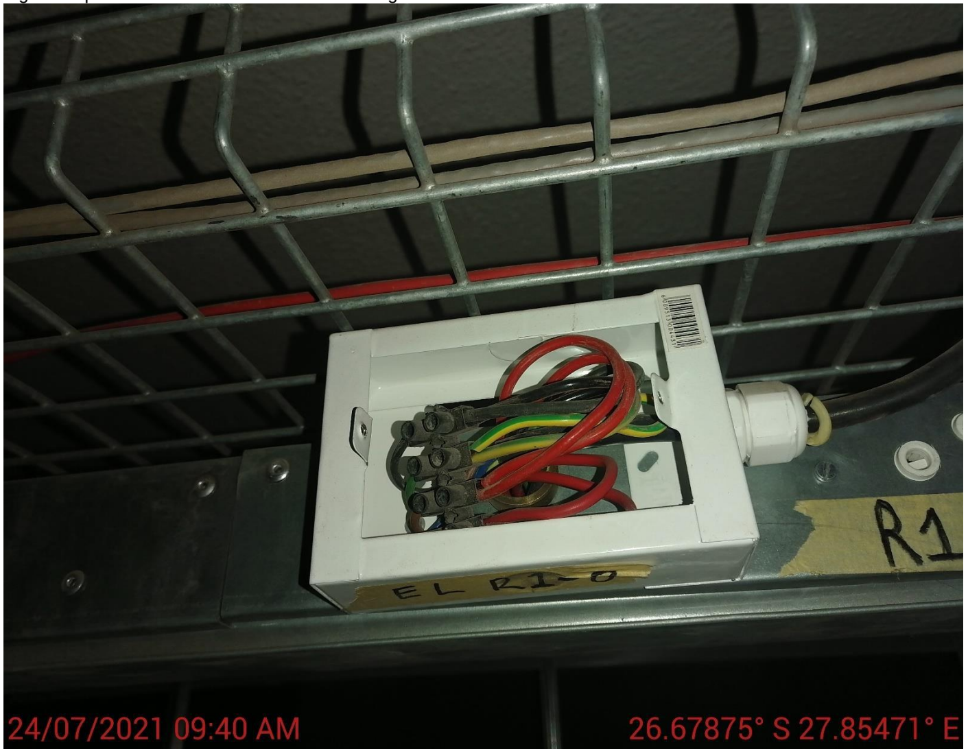
Fig 23 - Open Junction box – Tea Kitchen ceiling Void
