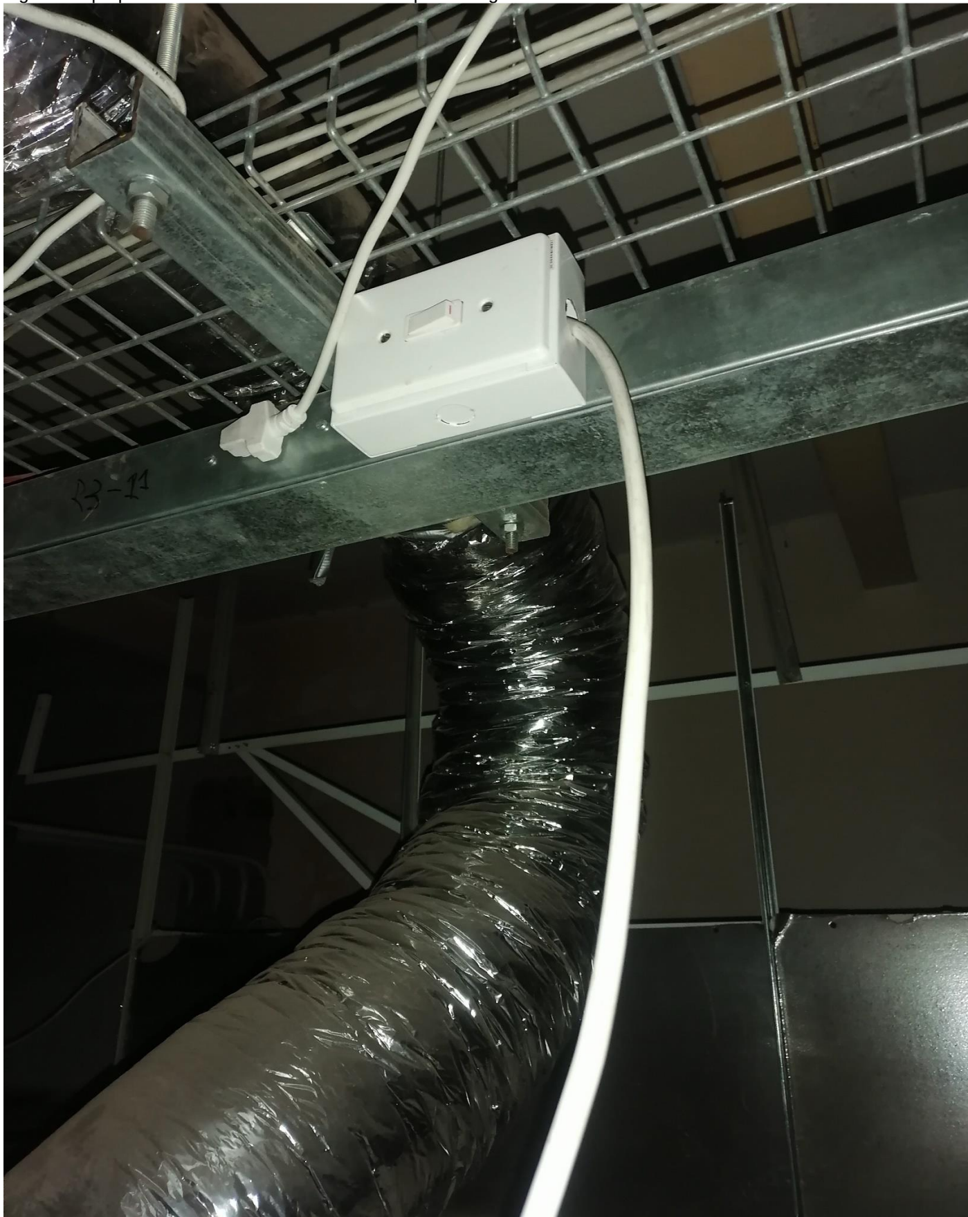
Fig 26 - Improper Cable termination – without compression glands
