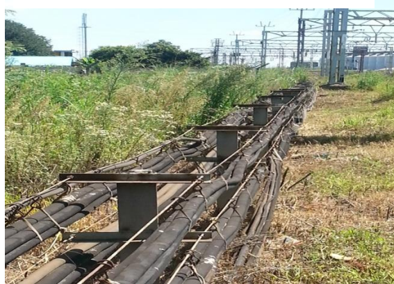
Figure 3 Vegetation poses fire hazard
