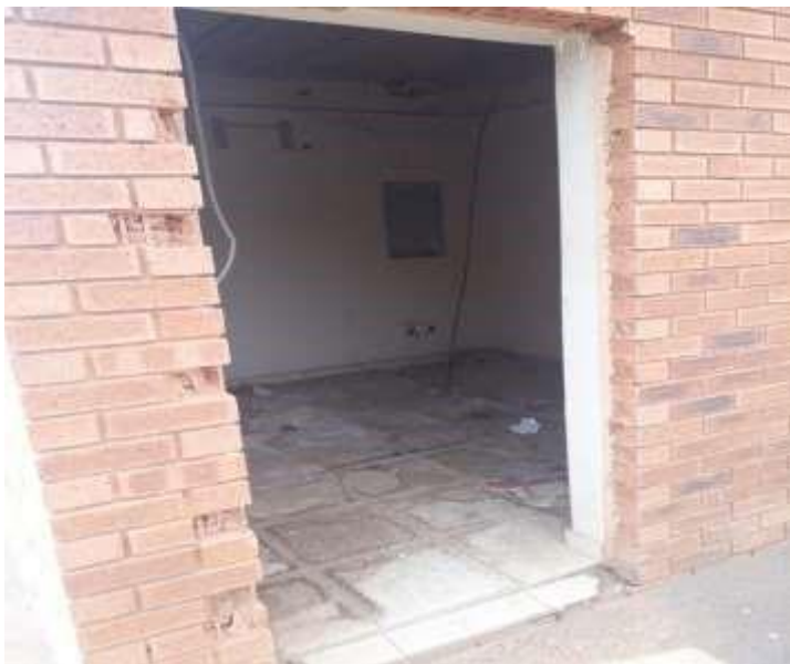
Picture 3: Vandalised structure at the station
