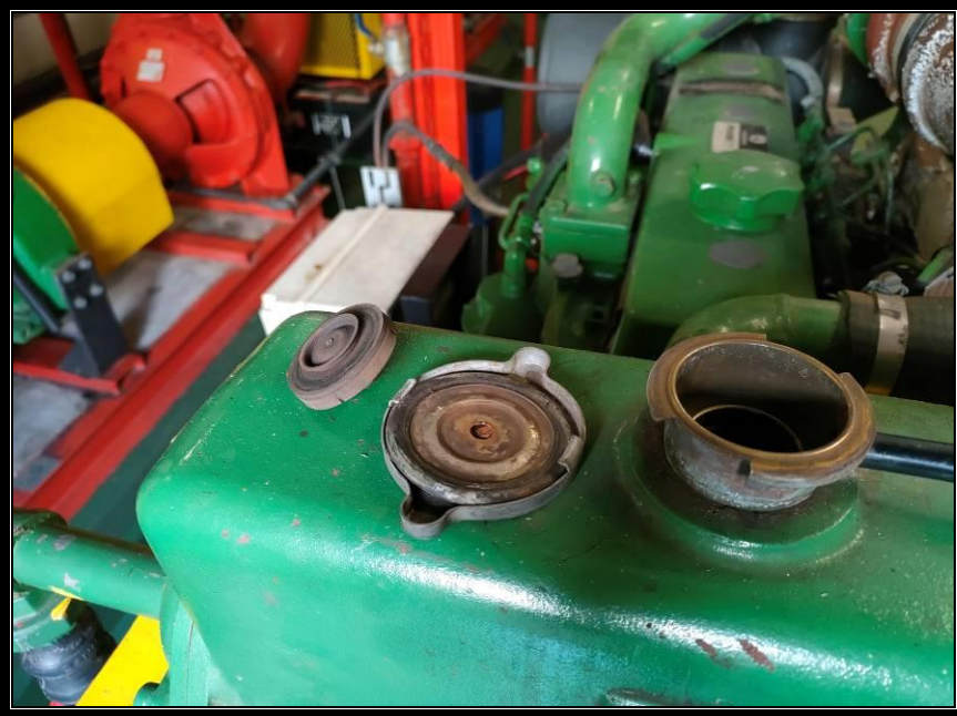
Figure 5: Cooling line Gauges
