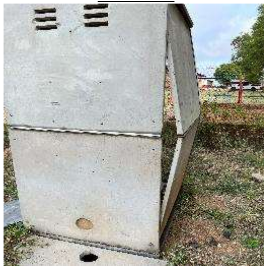
Collapsing amalooloo toilets
