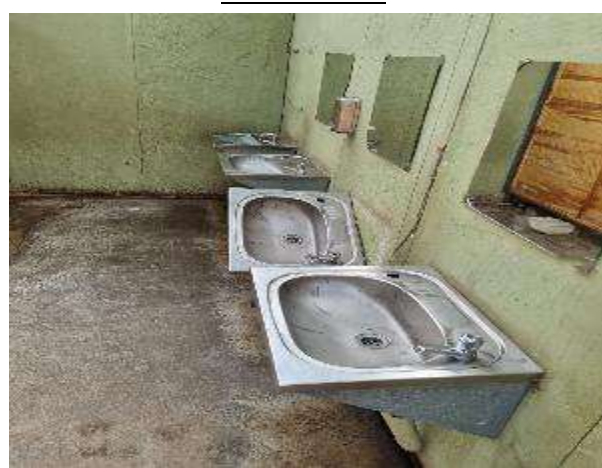
Damaged steel basins
