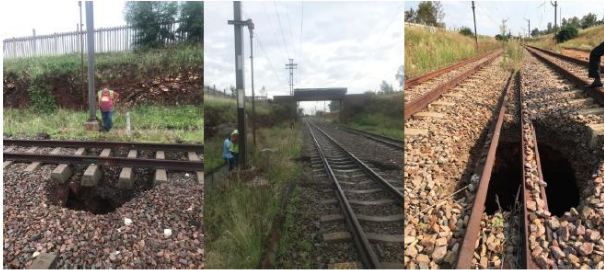
Figure 1: The re-occurrence of sinkholes in the Pinedene station area, WA Km 35 to 36
