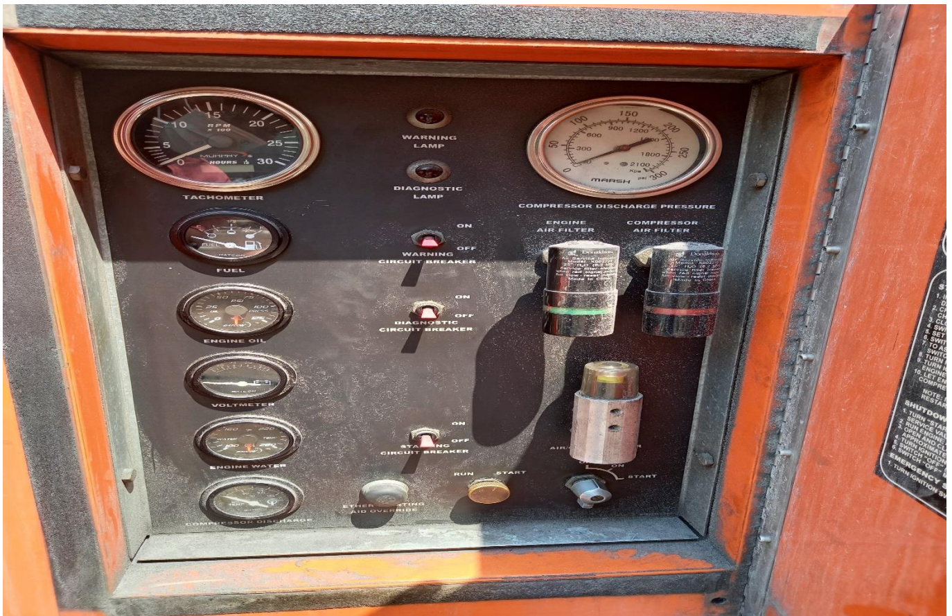
Figure 8: Diesel Compressor Local Panel
