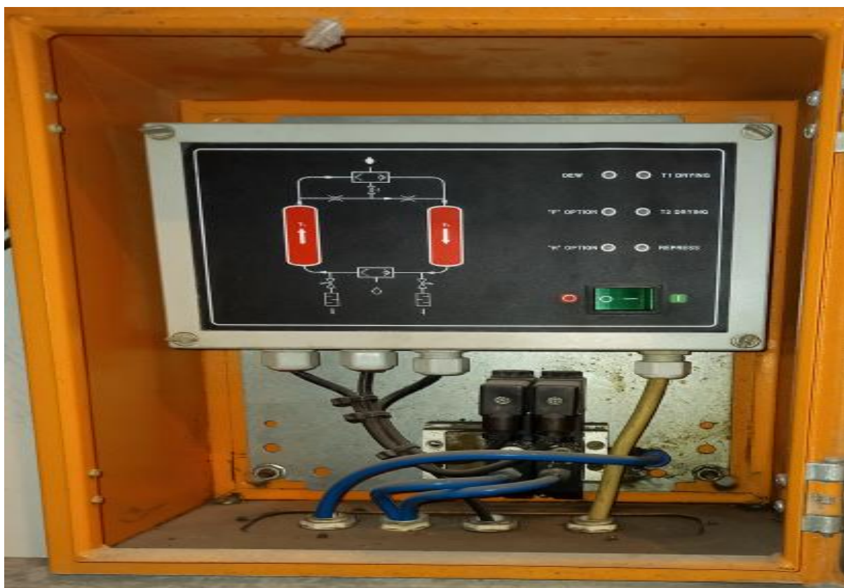
Figure 9: Diesel Compressor Local Panel
