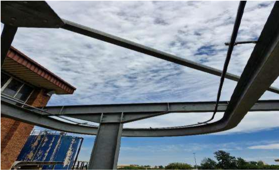
Figure 4: Damaged C-Track curve
