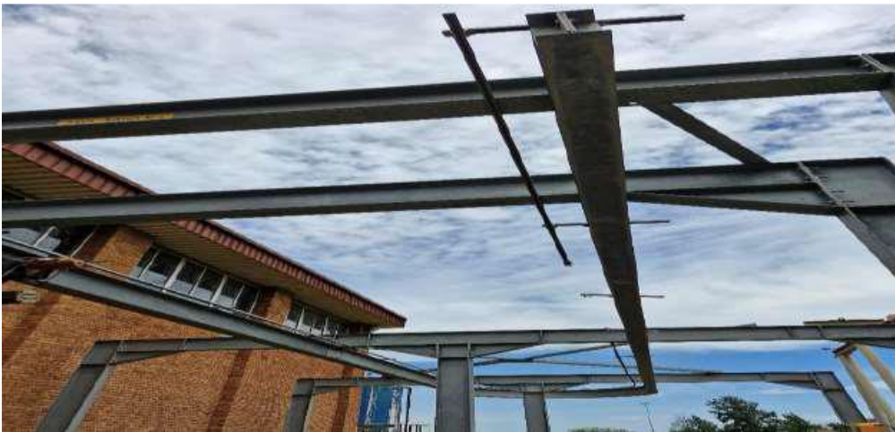
Figure 5: Missing C-Track portions
