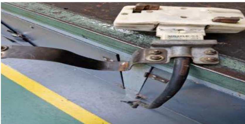
Figure 2: Damaged current carrier front view
