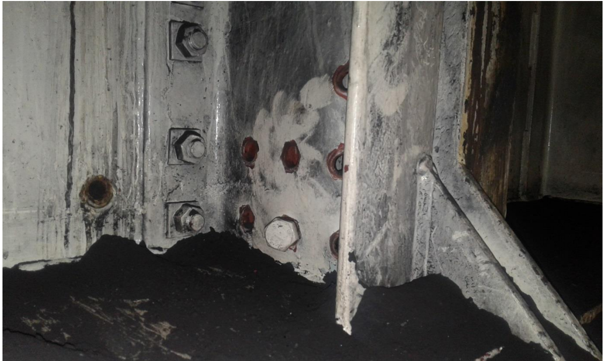
Missing liner connection bolts – TB1
