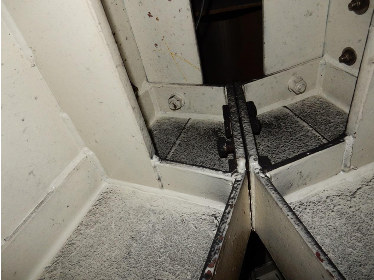
Loose hopper crotch connection bolt at TB1
