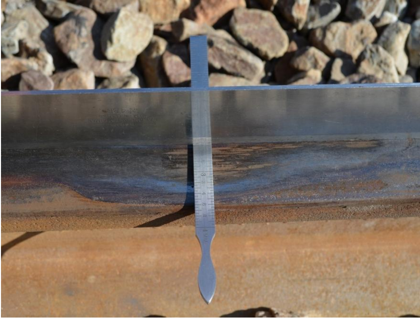
Figure 3: Measurement of Wheel-spin burns (skid mark).
