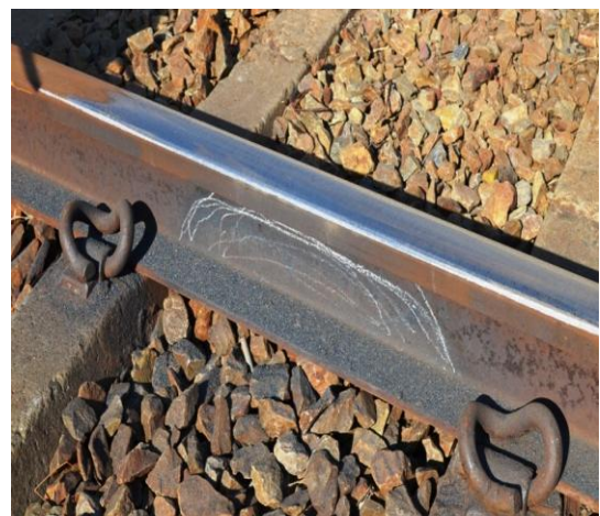
Figure 7: Wheel spin burns (Skid marks)
