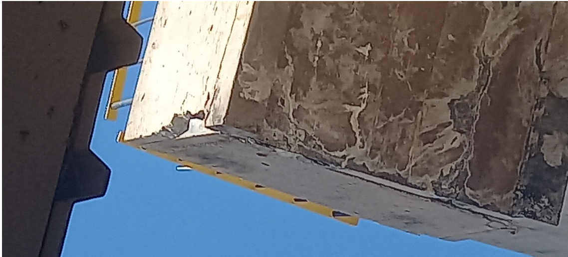
Figure 5 View of the cooling tower damage
