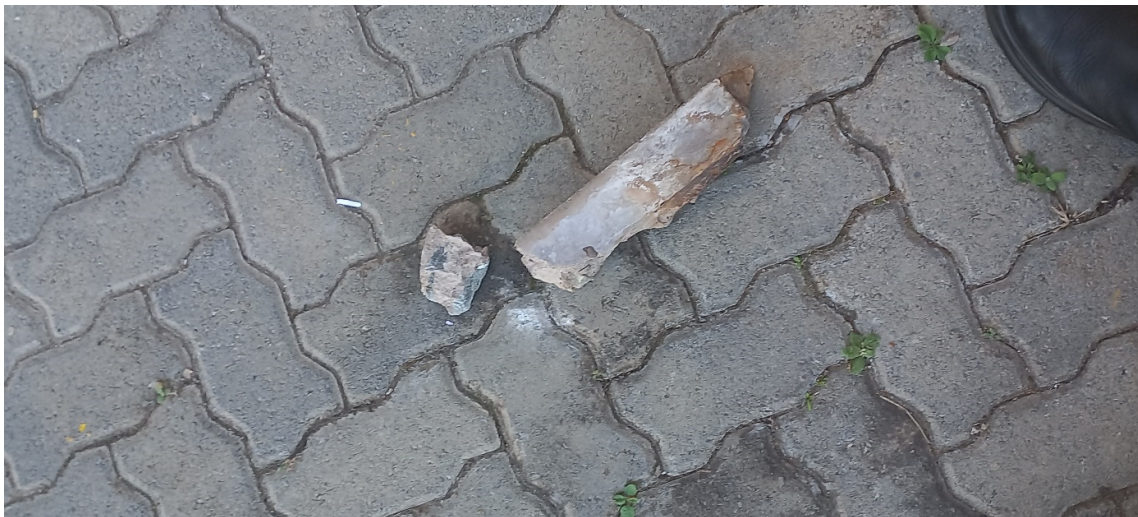
Figure 6 Piece of concrete that fell off the cooling tower
