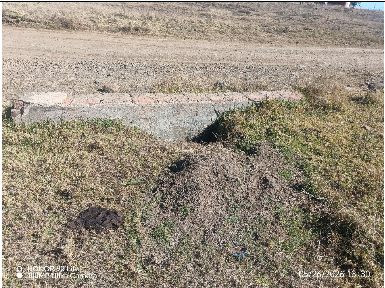
750mm circular culvert blocked
