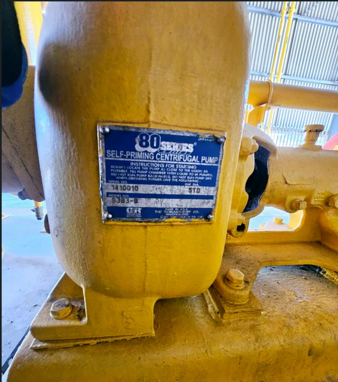
Inflow Pump Nameplate.jpg
