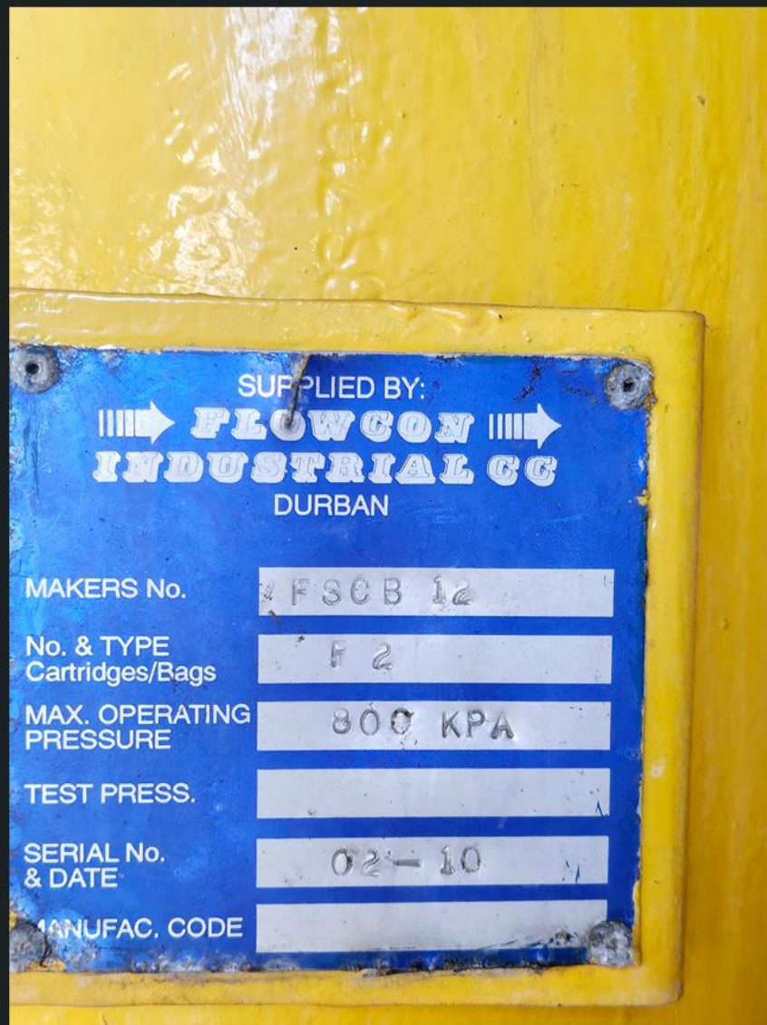
Inflow Valve Nameplate.jpg
