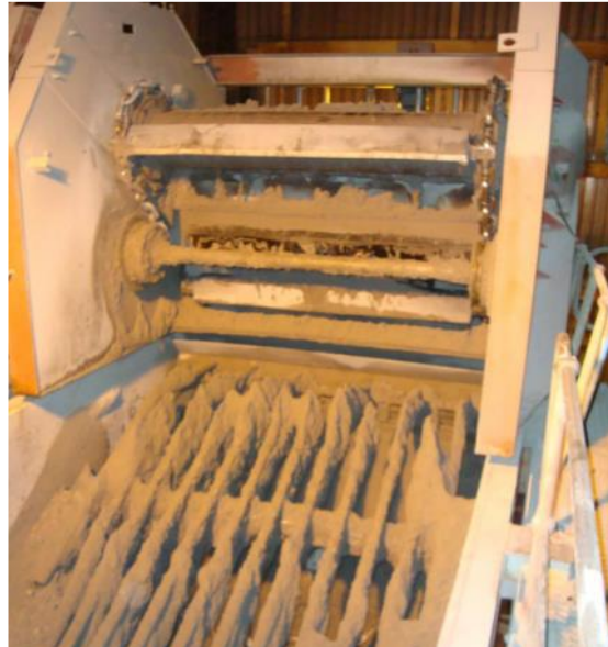
Figure 2: SSC chain and drive shaft assembly
