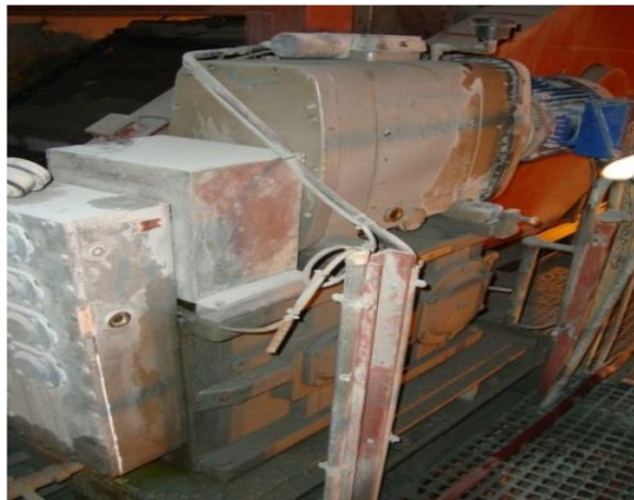
Figure 1: 3 gearboxes aligned to develop torque (Mechanical drive)
