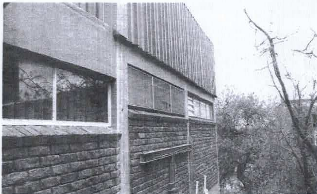
Photo 18: Bathroom window with metal mesh fly screen that need to be re-aligned. Noted: Windows without aluminium frames will not be re-aligned with metal mesh fly screens.
