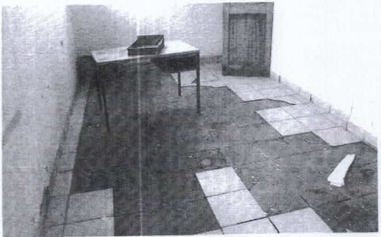
Photo 4: Lecture Room floor tiles that need to be removed and the similar or equivalent to OGrady's coprox 800/200 Epoxy to be applied.
