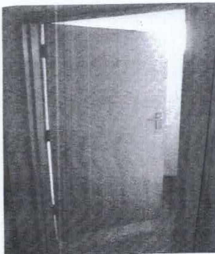
Photo 8: Bathroom wooden door that needs to be sanded down and repainted with white enamel paint (similar or equivalent to OGradys undercoat).
