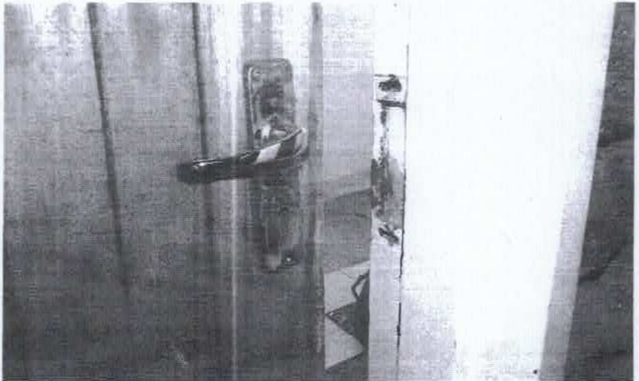
Photo 20: Wooden Door with 3 lever lock and striker plate that needs to be replaced, (2 keys need to be supplied)
