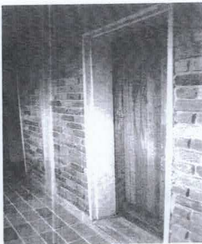
Photo 7: Dormitory Wooden Door that needs to be sanded down and re-varnished with metal frames that needs to be repainted with enamel paint (similar or equivalent to OGradys undercoat).
