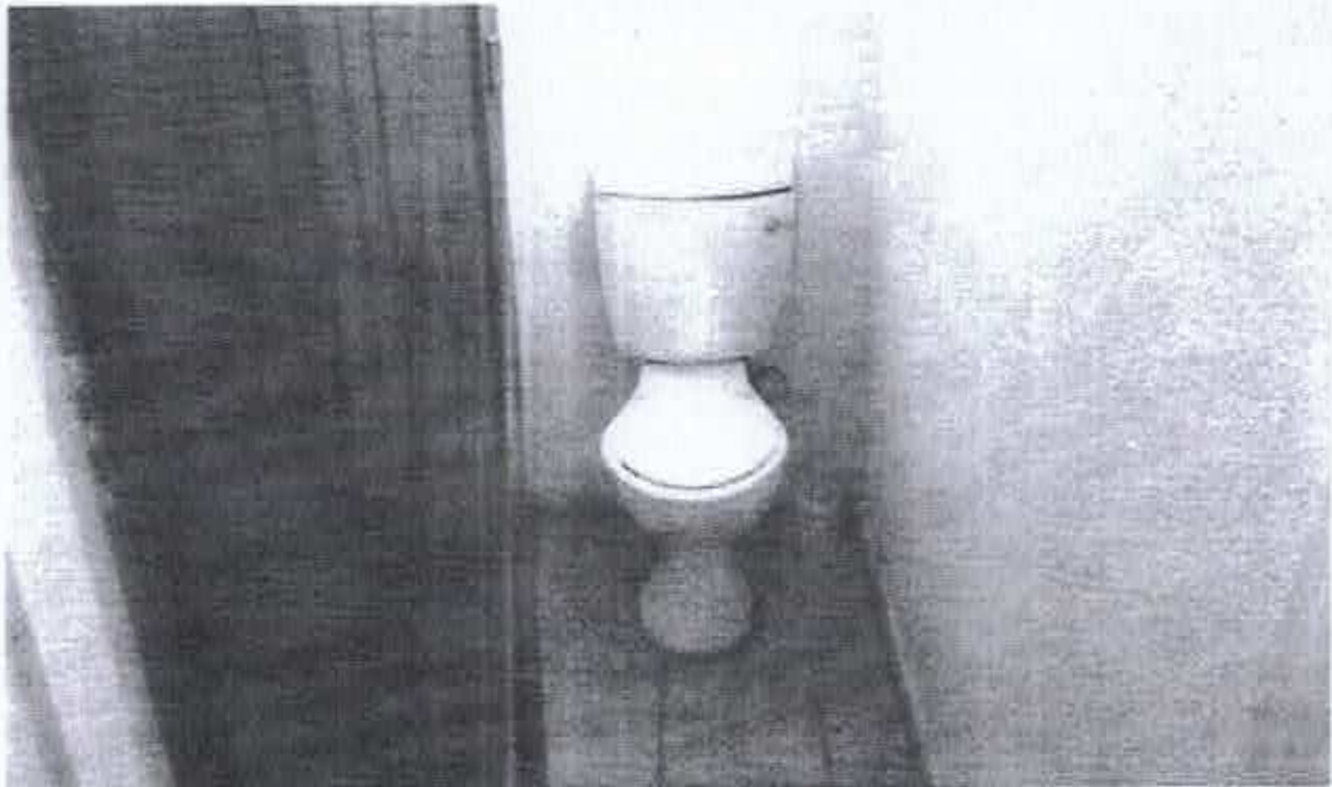
Photo 14: Bathroom Toilet with cistern kit that needs to be replaced in D3 with a Universal cistern kit. One (1) toilet seat to be replaced with a Universal plastic seat, white of the top floor of D5 accommodation block.
