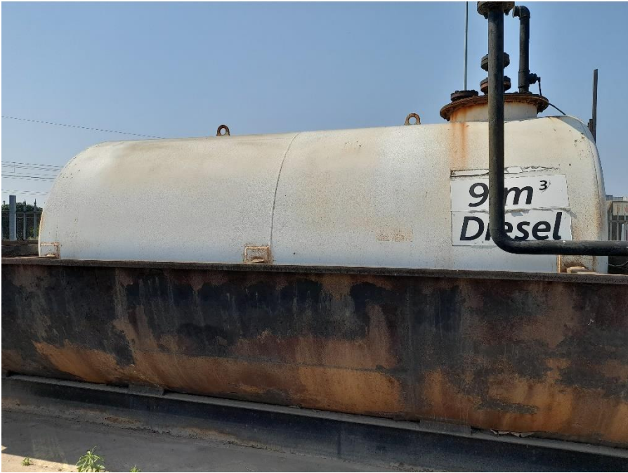
Diesel storage tank
