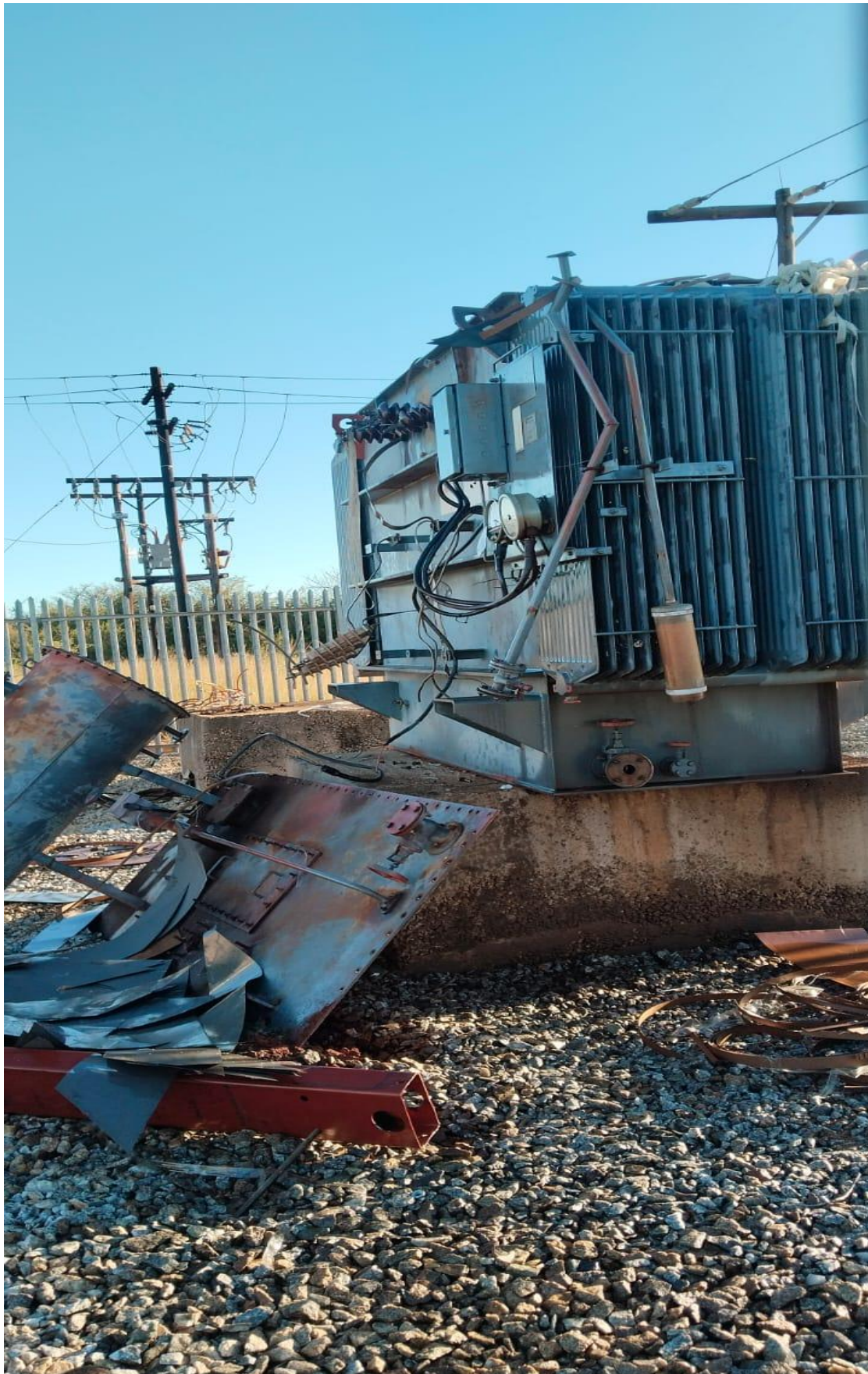
Picture for the 5MVA Transformer Serial Number 73151 located at located at the Nantes Substation .
