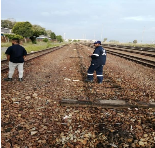
Fig 2.1: Missing sleepers and vandalised track
