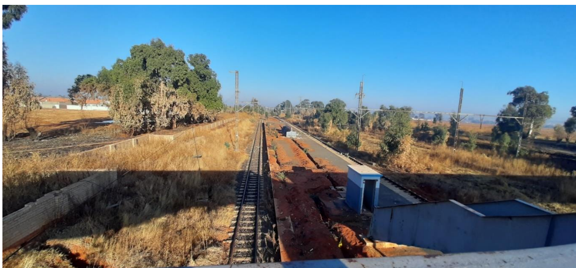
Dug Up Platform Surfaces to be resurfaced and the half brick wall to be extended too the height specified in the scope of work in-line with PRASA security requirements.
