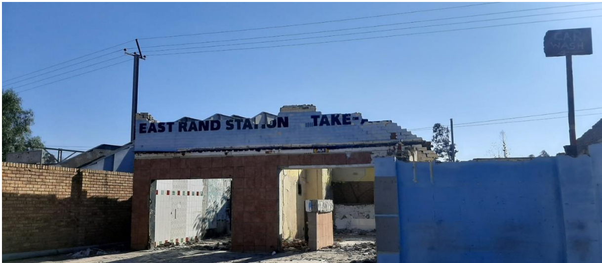
Station Entrance old take away shop – To be demolished and space to be used as the new Ticket Sales Office
