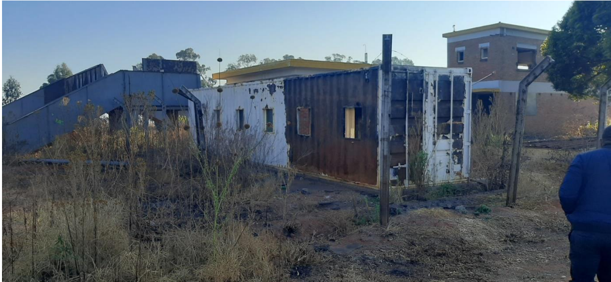
Burnt container Ticket Office – Container to be reused where possible as part of the ABT T/O facilities. This container will be inspected for durability and be repurposed if possible.
