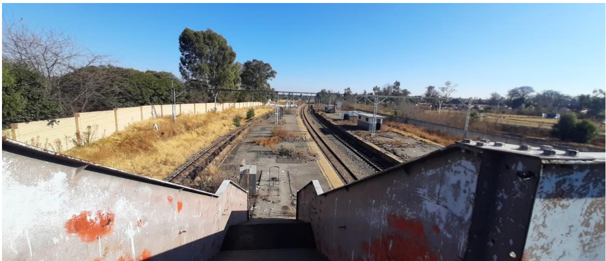
Vandalised platform ticket verification points – To be rehabilitated and ABT points to be implemented
