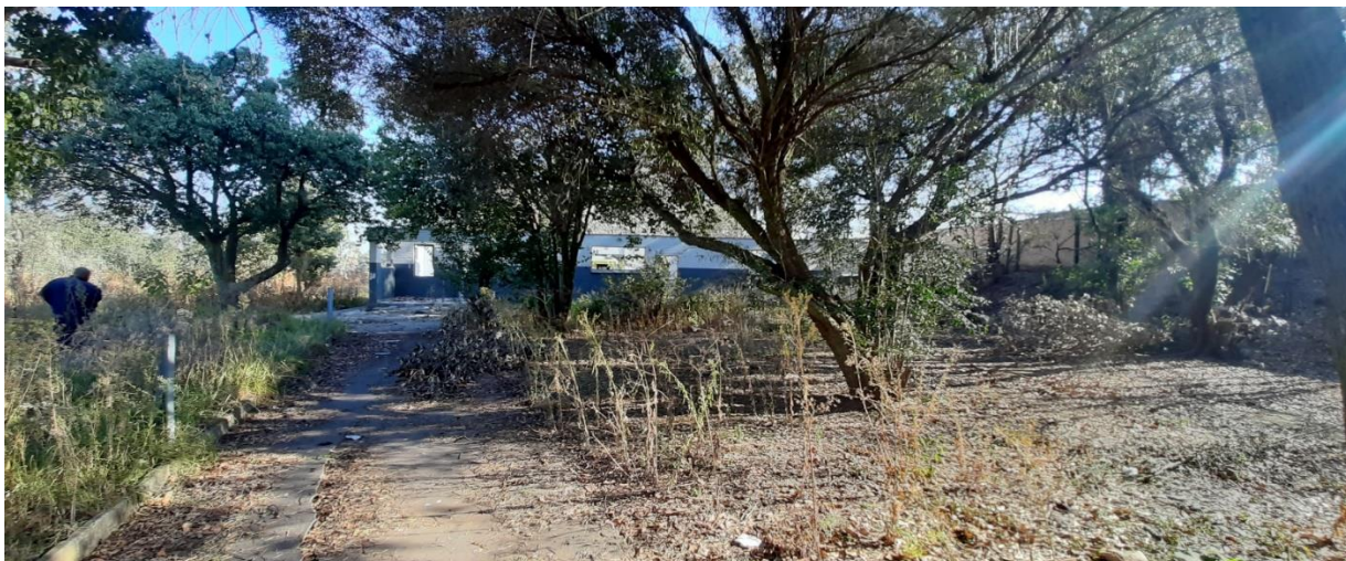
Vandalised Ticket Office in the bushes – To be demolished and area cleared out.
