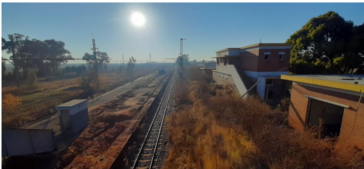
Dug up Platform Surfaces to be resurfaced – Scope of work shall provide details
