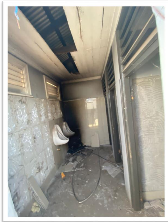
Vandalized toilet facilities.
