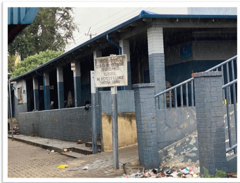
Aging building. Paint peeling off walls.
