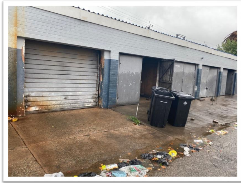
Aging building. Rust on garage steel doors, and paint peeling off walls.
