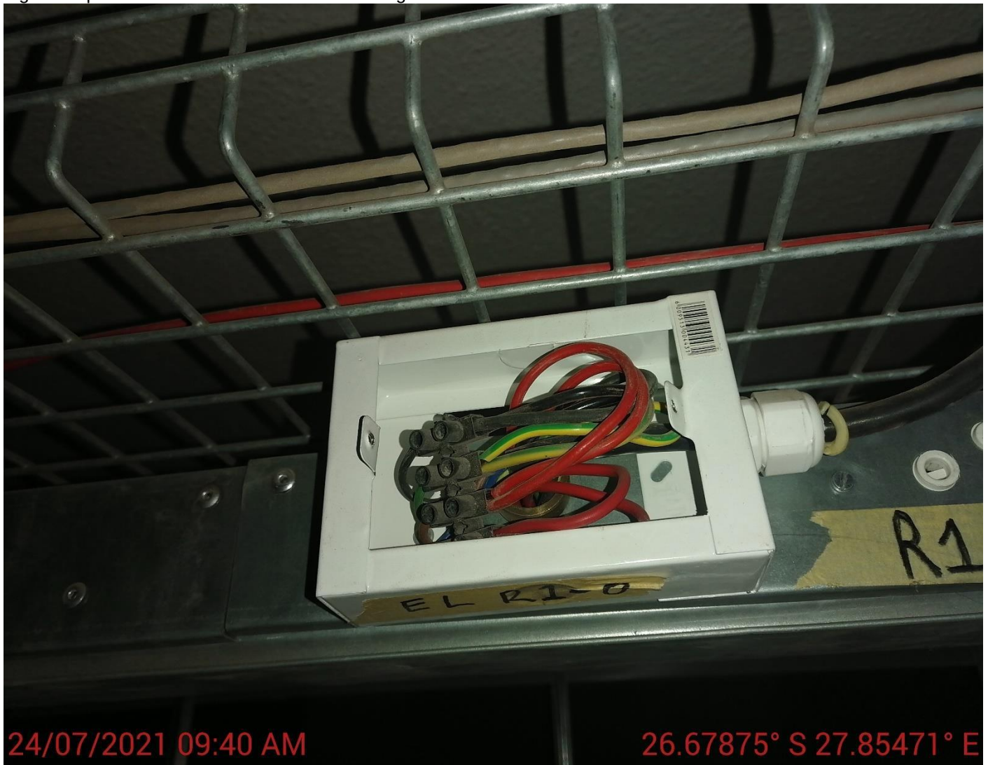
Fig 23 - Open Junction box – Tea Kitchen ceiling Void
