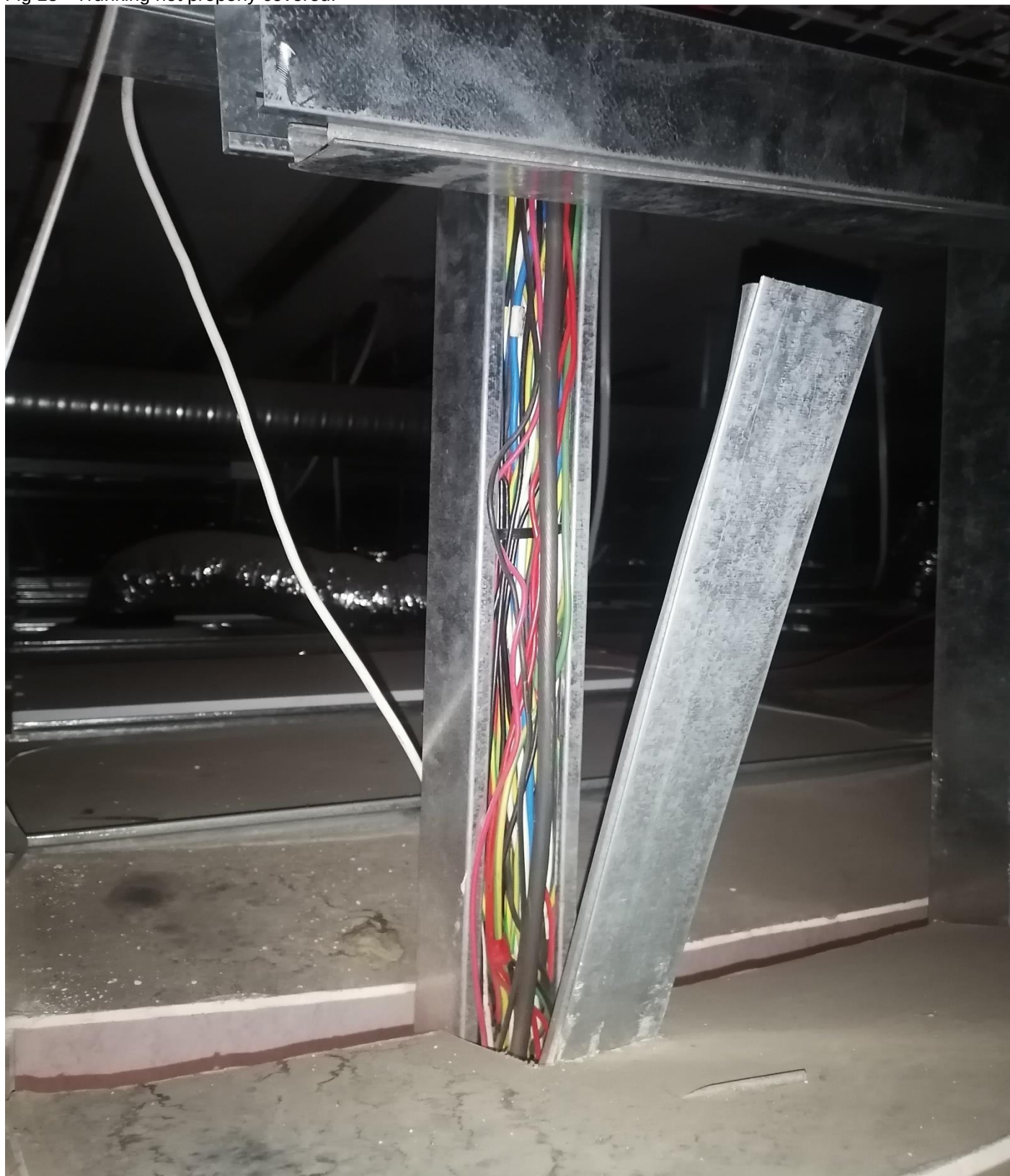
Fig 15 - Trunking not properly covered.
