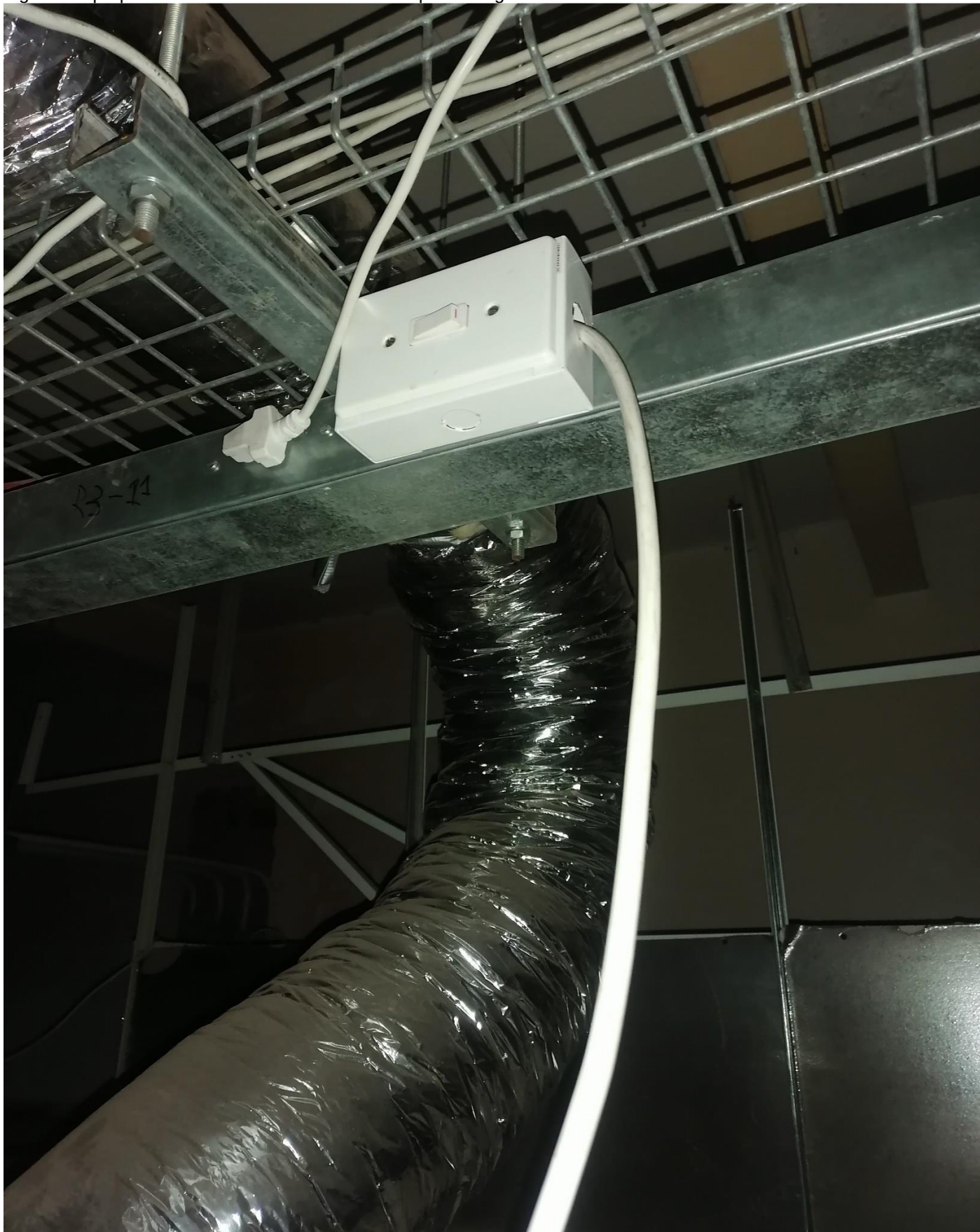
Fig 26 - Improper Cable termination – without compression glands
