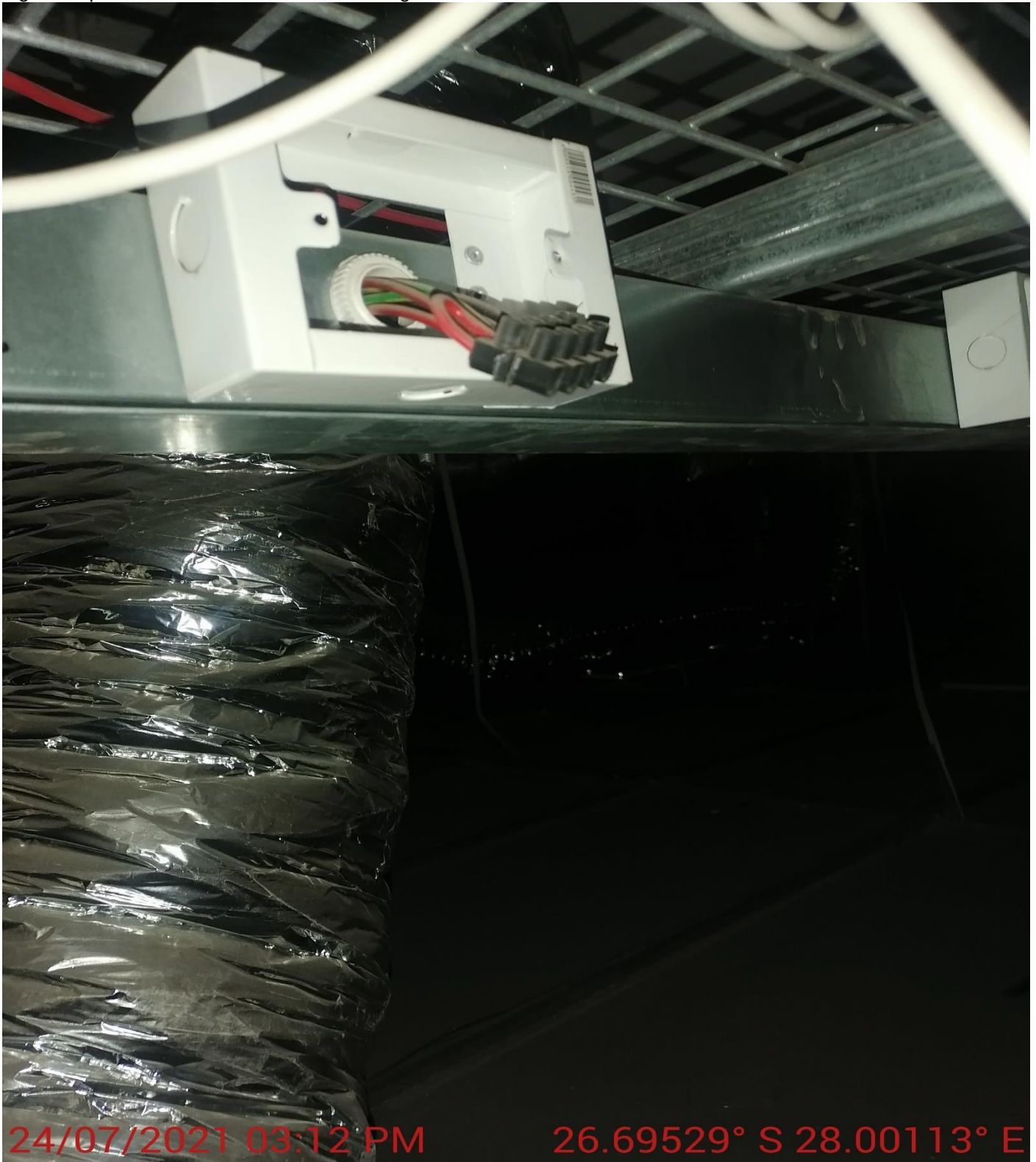
Fig 19 - Open Junction Boxes inside the ceiling void
