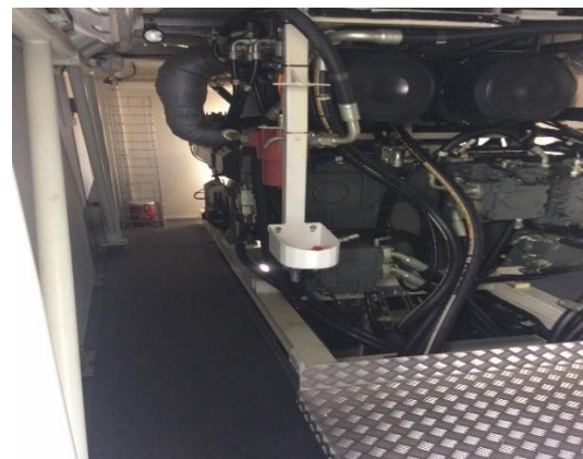
Figure 2(d) Engine Compartment
