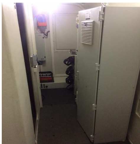
Figure 2(e) Electronic room
