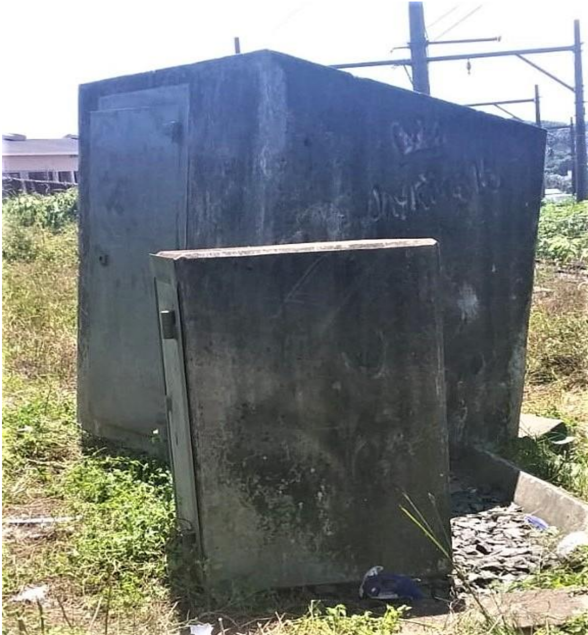
Figure 1: Concrete Cases at Greenwood Park
