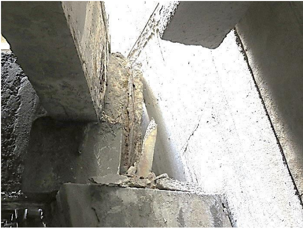
Figure 5: Cracking and spalling at beam corbel connection Attack
