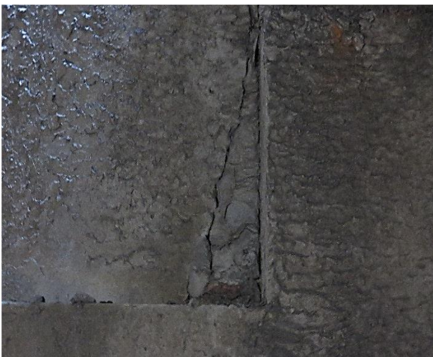
Figure 3: Cracking at beam edge Cracking
