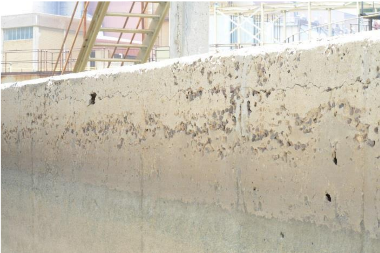
Figure 7: Pond internal walls cracking.
