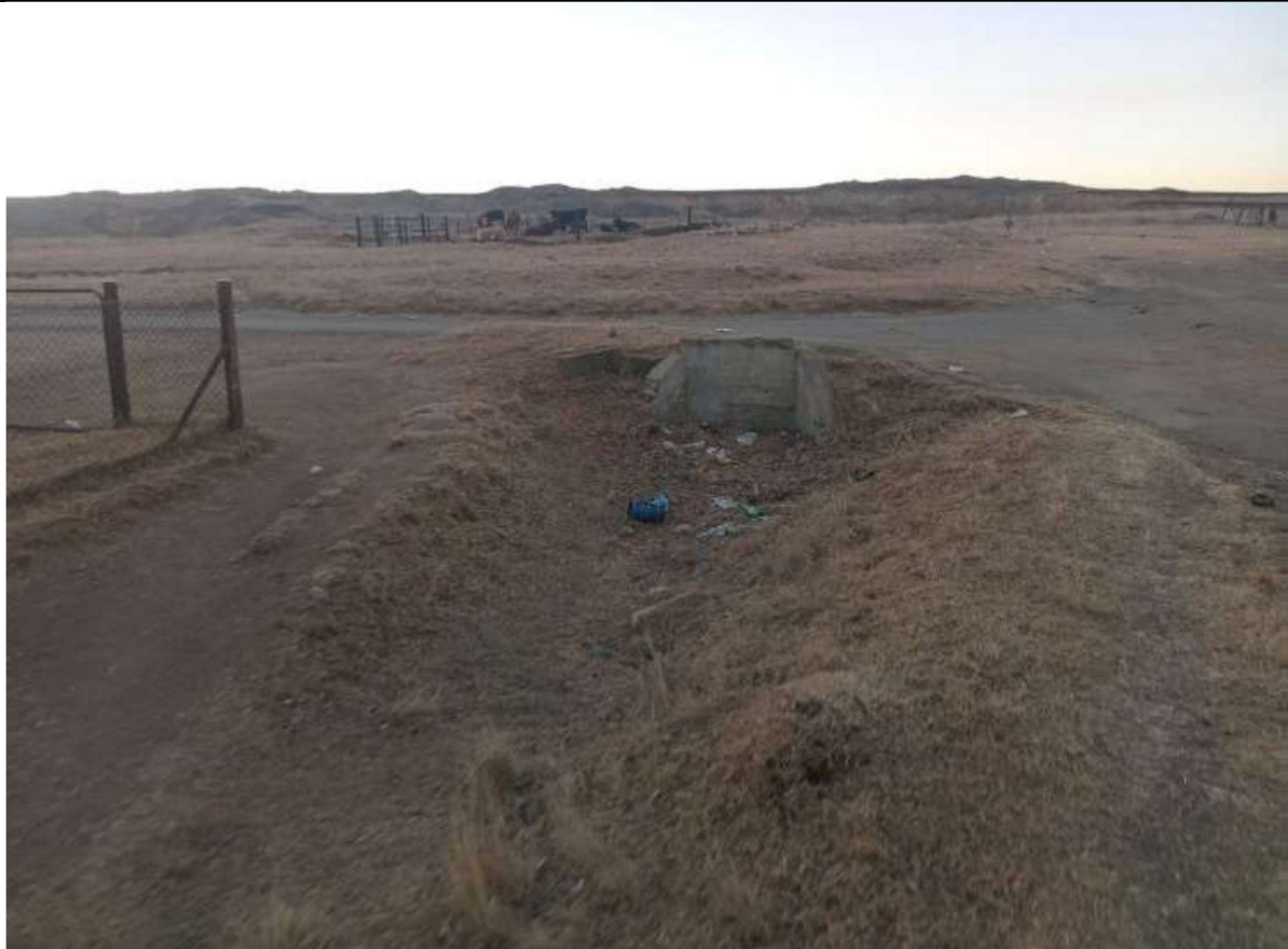
Block/clogged Existing Culvert
