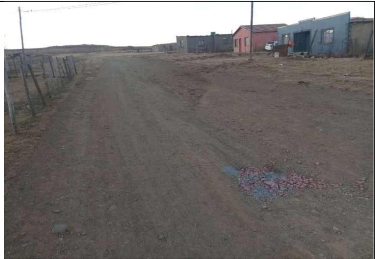
Damaged Existing Road way
