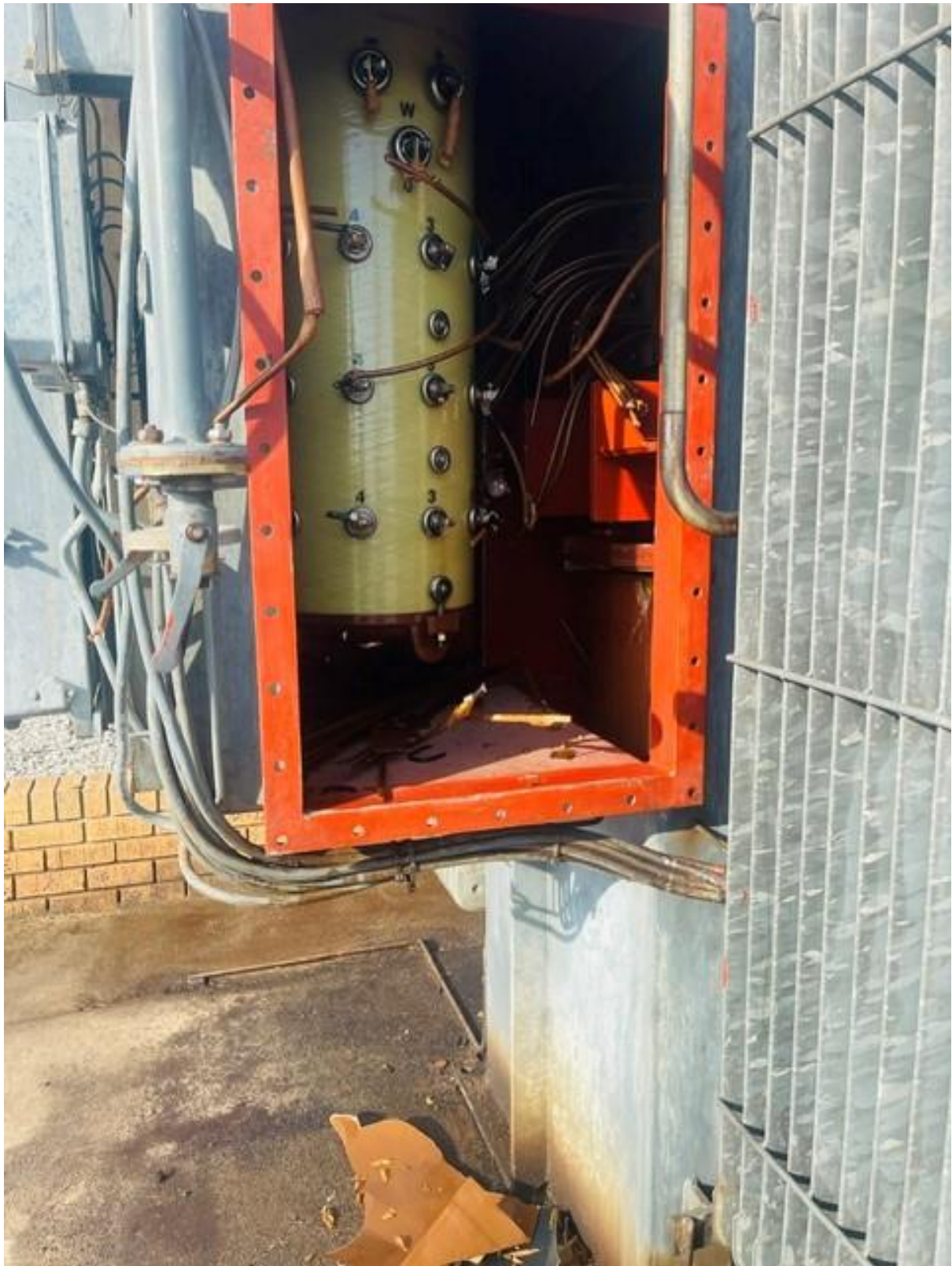
Picture of Ga-Maja 5MVA Vandalized Transformer, Serial Number T-2199 39-112
